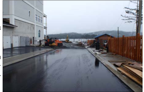
Construction of the Public Boat Launch is well underway and is anticipated to be completed by Summer 2011.
